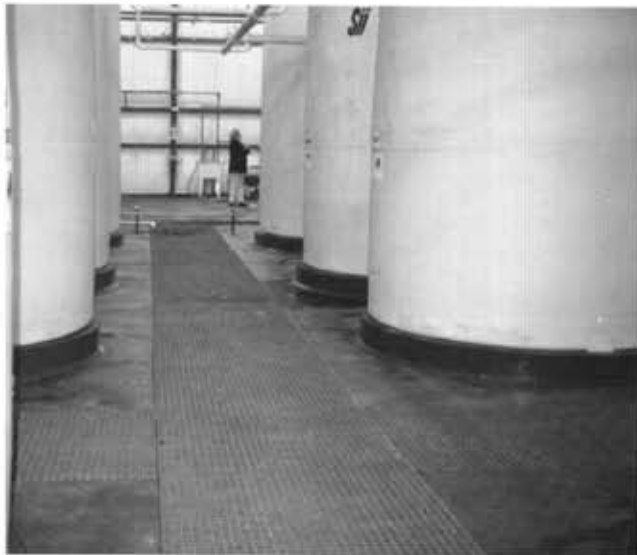
The Exide Battery Plant in Manchester, Iowa installed corrosion resistant DURAGRATE® around its tanks of sulfuric acid.
